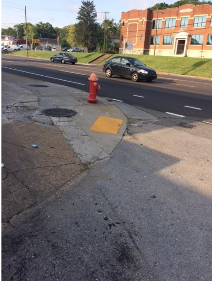
Non-Flush Curb Ramp Transition
