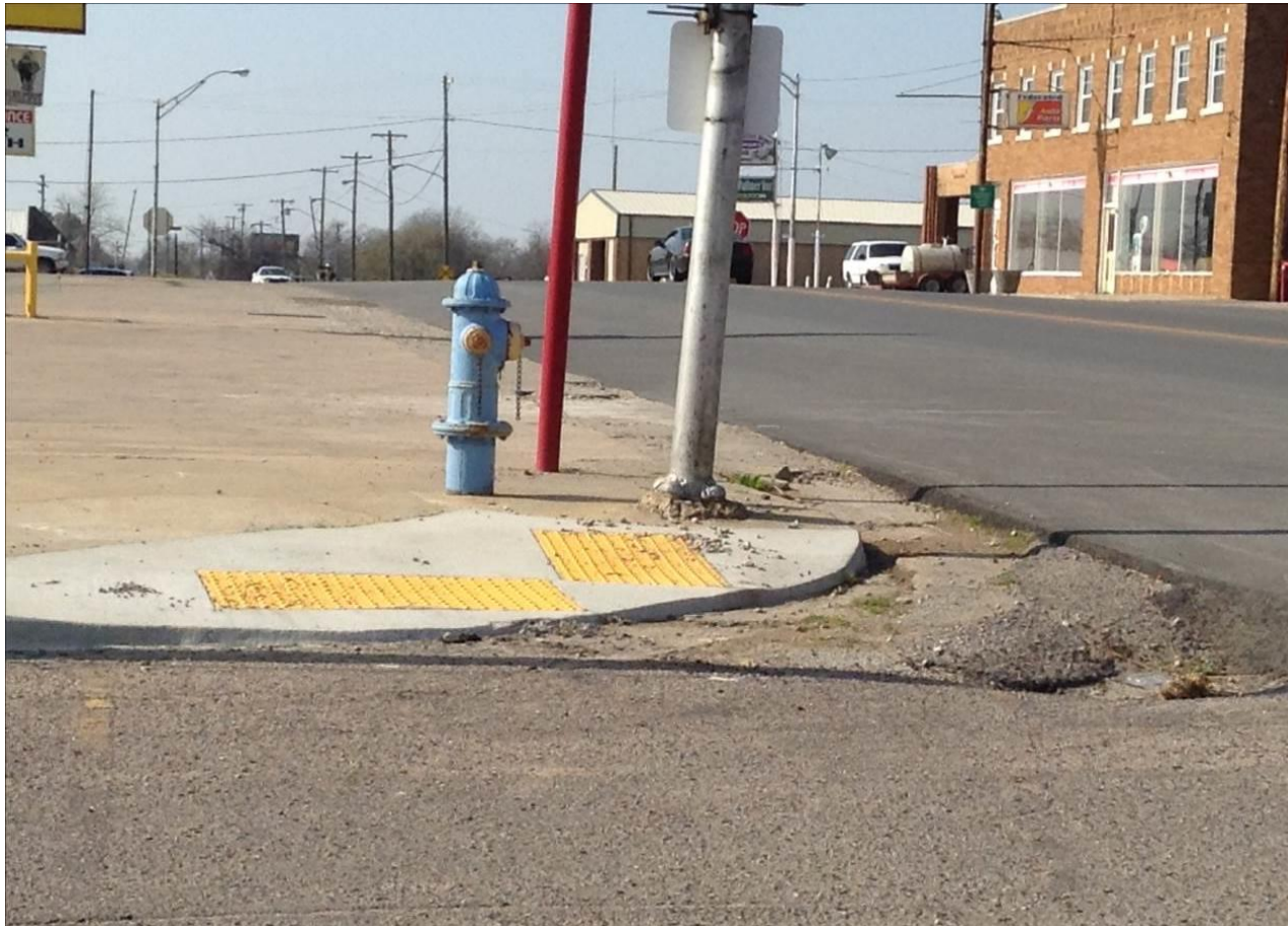
Non-Flush Curb Ramp Transition
