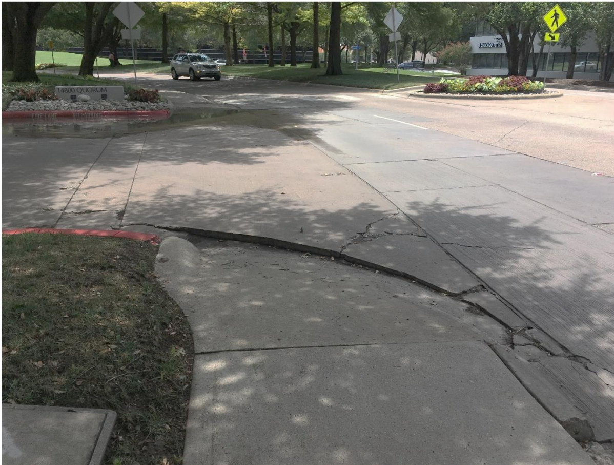
Non-Flush Curb Ramp Transition
